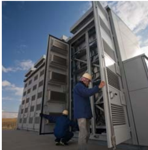
A 7.2 megawatt-hour battery in Minnesota.
